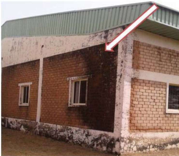
B.1(b): The vertical wall shown with a pointer has dark patches as a result of undrained water from the cladding
