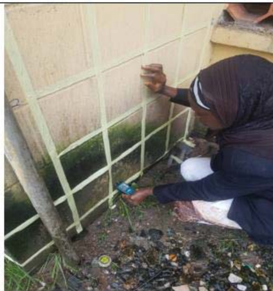
Plate D: The identified wall showing symptoms of rising damp
