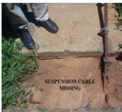
Figure 11: Suspension cable being attacked by corrosion and one of the cables already snapped
