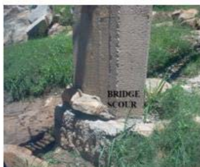
Figure 9: Scoured support bases
