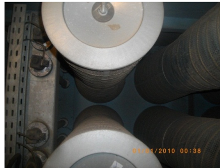
Figure 1. Pulse filters before cleaning
