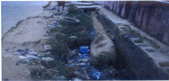
Figure 2: Showing a poorly maintained drain (Olukanni et al. , 2013)
