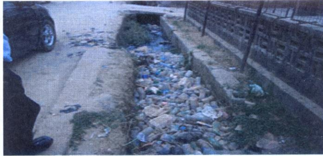
Figure 1: blocked drains as a result of abuse of drains with waste deposits (Olukanni et al. , 2013)
