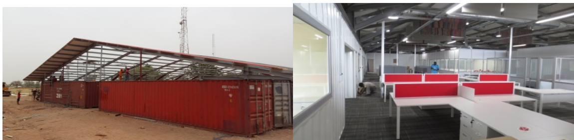
Figure 1 Plates showing the containers and the roofing carcass and the interior (workstations) when completed
