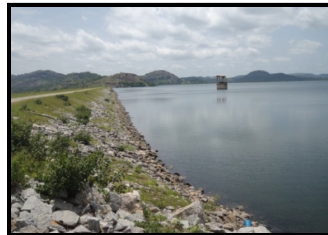
Plate V. Upstream of the Lower Usuma Dam showing the Dam Embankment, Reservoir and Intake Tower Structure
