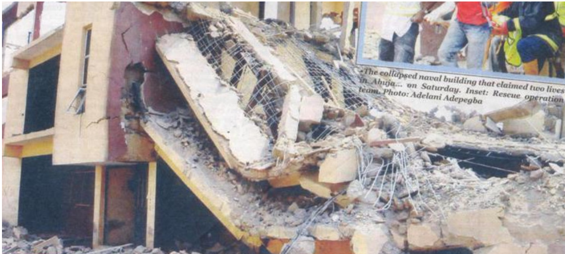
Figure 3: Building collapse as result of engagement of quacks/non-professionals (Source: Sunday Sun Newspaper' of January 29, 2012)
