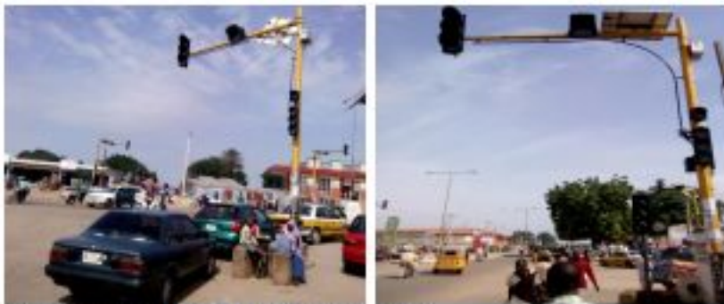
Plate 2a & b: Present condition of traffic light in Minna
