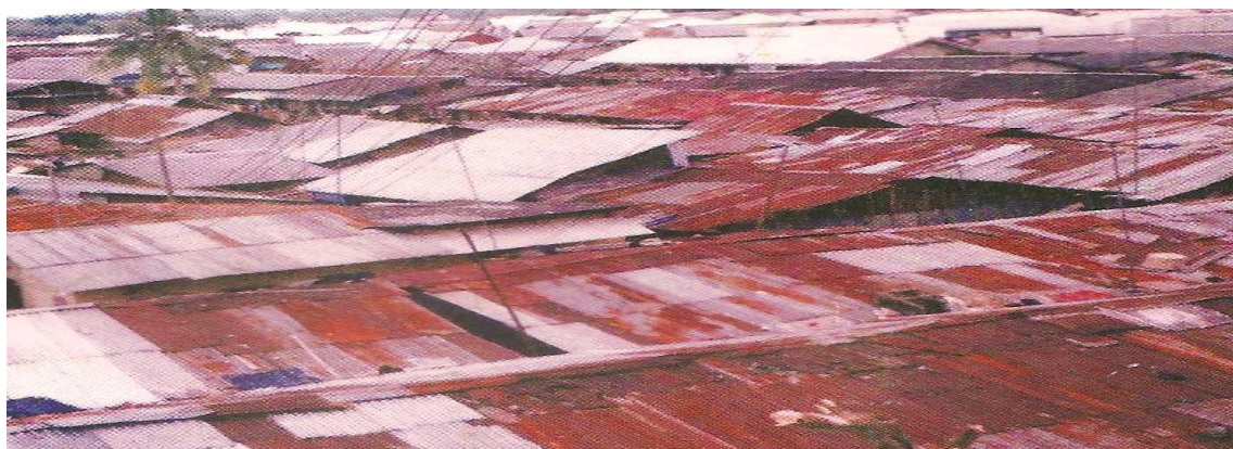
Plate 2. Cluster of zinc roofs with various degree of rusting/caving-in
