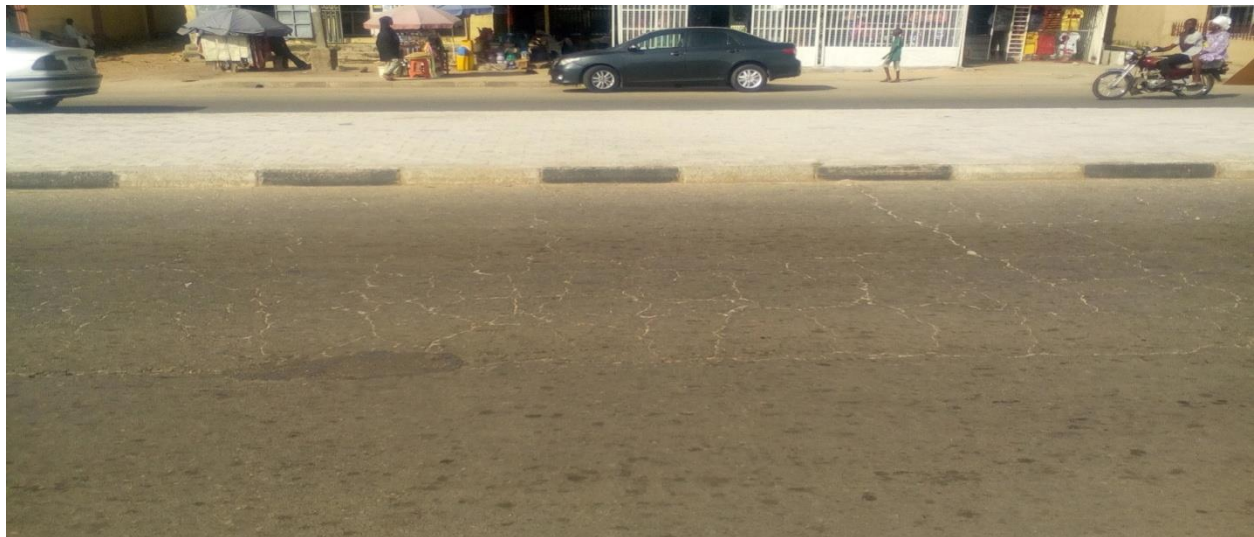
Plate I Alligator cracks along Bosso Road
