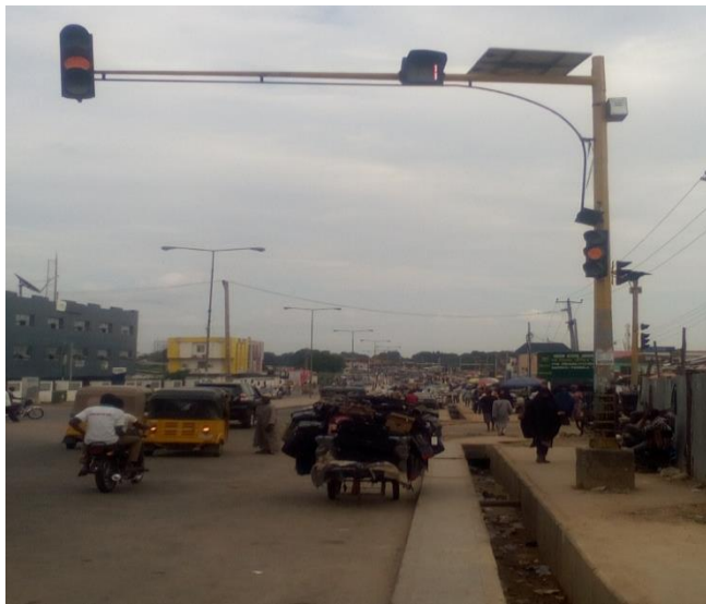
Plate V Damaged Traffic Light along Bosso Road
