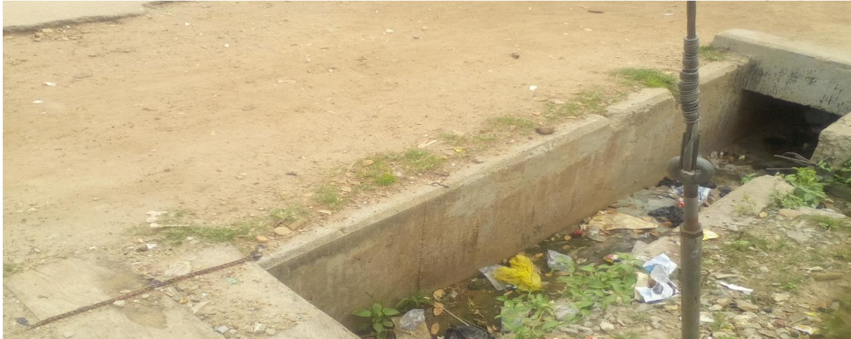
Plate IV Blocked Drainage along Stadium Road
