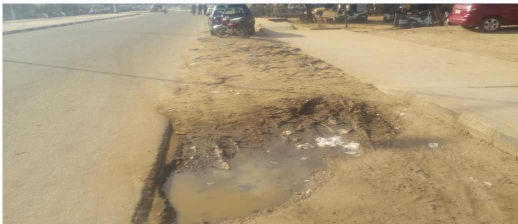
Plate II: Condition of Road Shoulder on the Bosso Road
