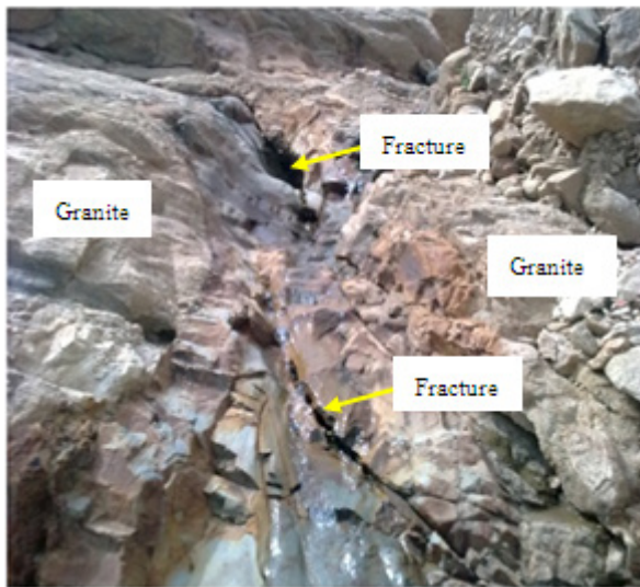
Figure 4. Photograph of fractures that permit water to percolate and cause weathering and weakness of the rock unit
