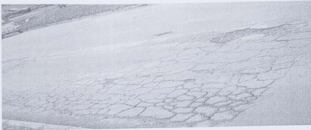
Figure1 A failed portion of the studied road
