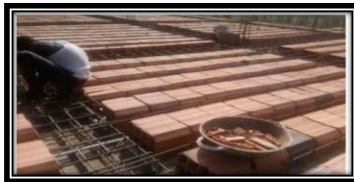
Plate 10: Shows hollow construction bricks use in the construction of first floor of a five bedroom Duplex Apartment, in Ibadan, Oyo state Nigeria. . Source: Author field work (2021)
