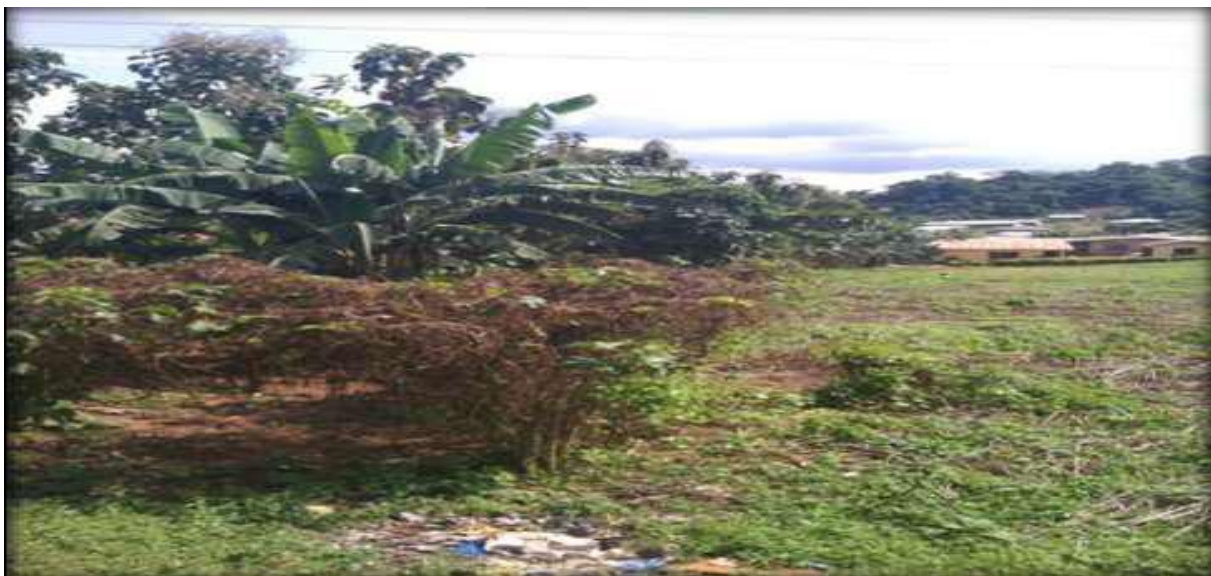
Plate 1: Farmlands being cleared and prepared for building construction around the study area
