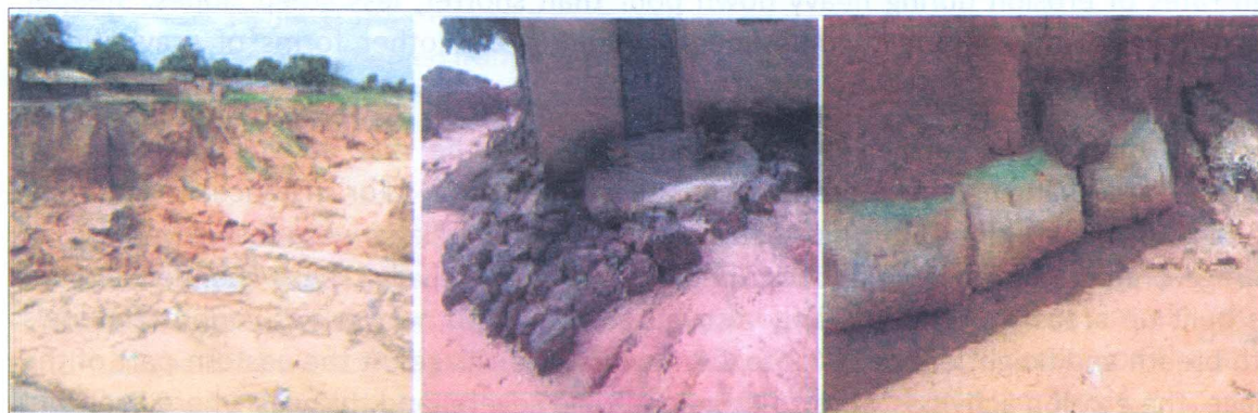
Figure 3. Gully erosion and sandstone used as foundation embankments in Rafingora.
