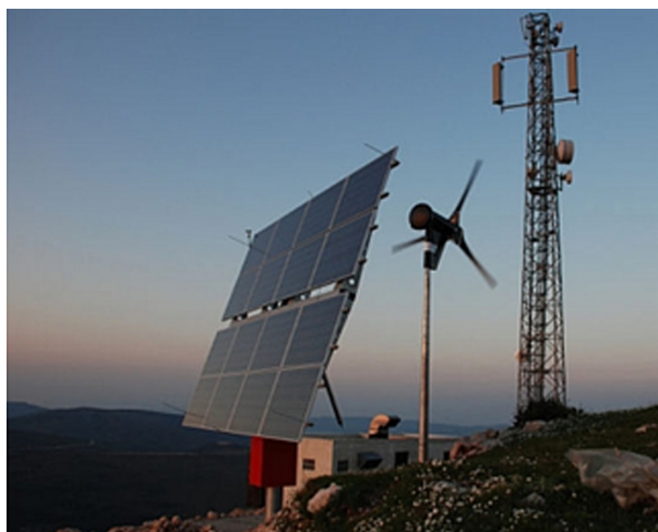
Figure 1. Off-grid hybrid PV–wind–diesel powered mobile base station.
