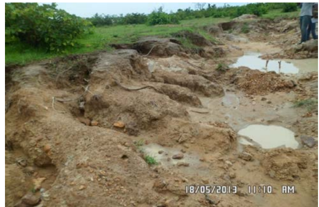
Figure 7. Photograph showing a new stream channel being formed as a result disrupting of the old channel by erosion.
